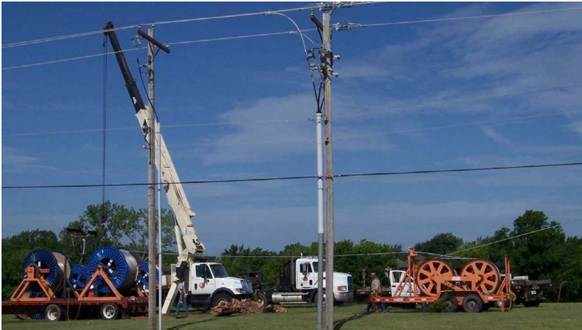
Three to One Ratio Between Tensioner and First Structure
